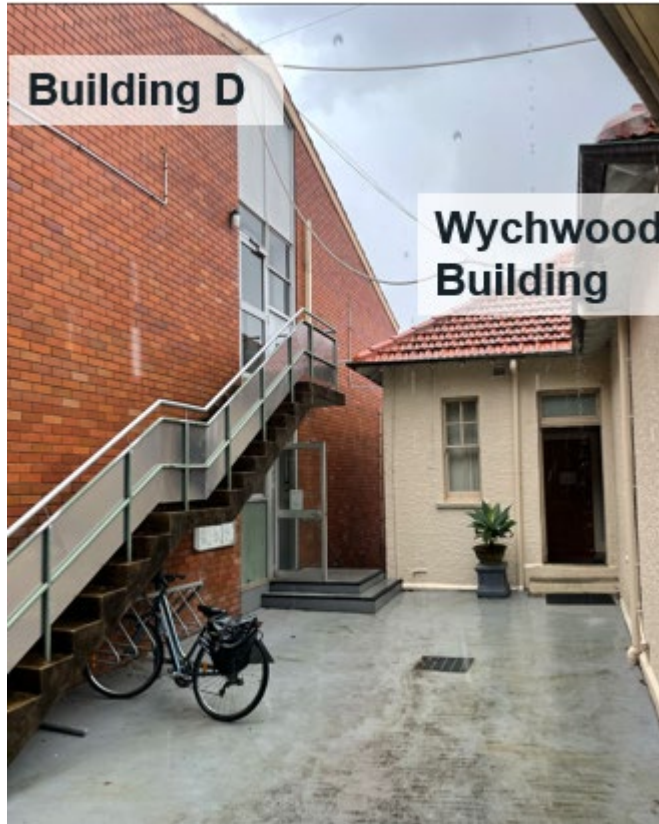
eastern elevation of Building D and south-western elevation of Wych Wood Building
